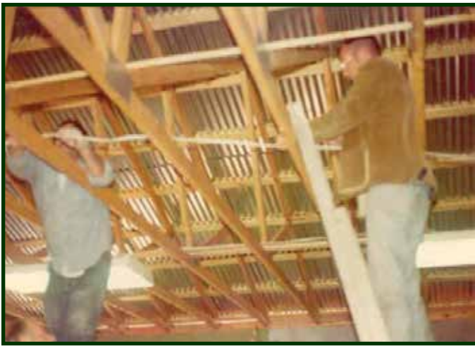
First DTCDC President Jim Walsleben works on the facility's electrical installation in December 1975.
